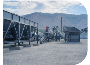
Drum Mix Plant with RAP System
